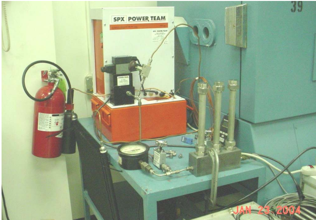
Photograph No. 11. Typical Hydraulic Impulse Mechanical Setup
